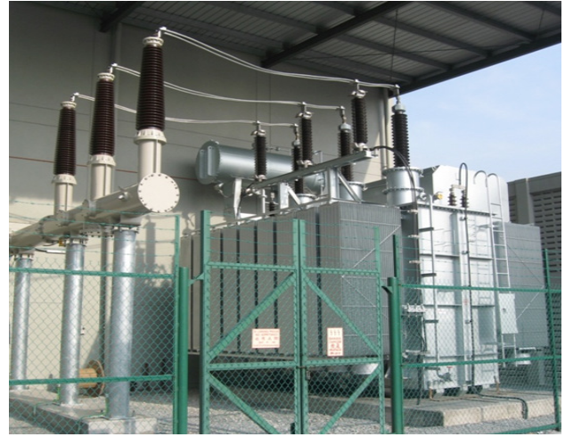
132/33kV 90/125MVA Power Transformer
